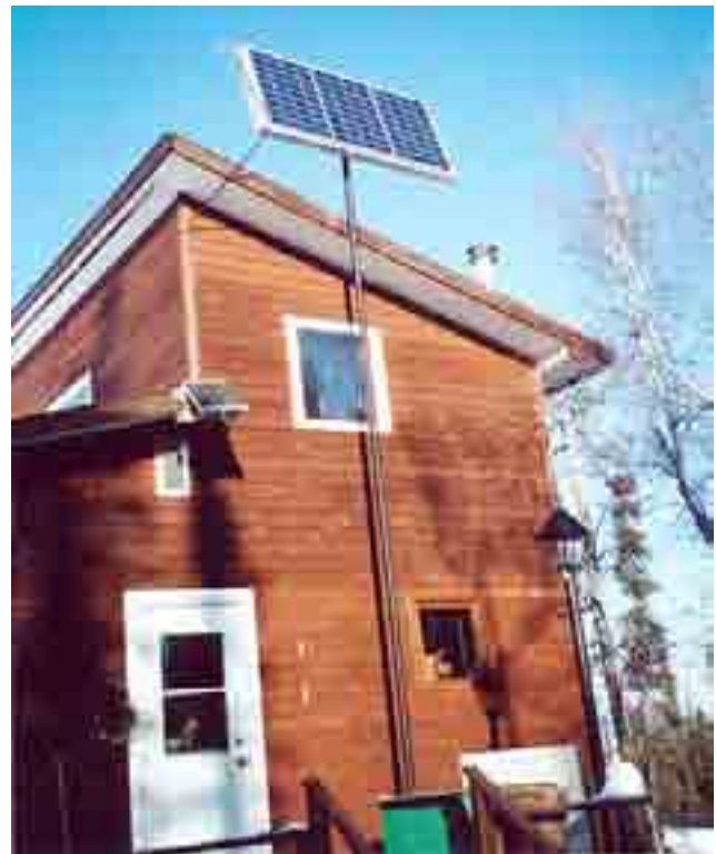
Solar Array for a Local Home Owner - RWED Photo
